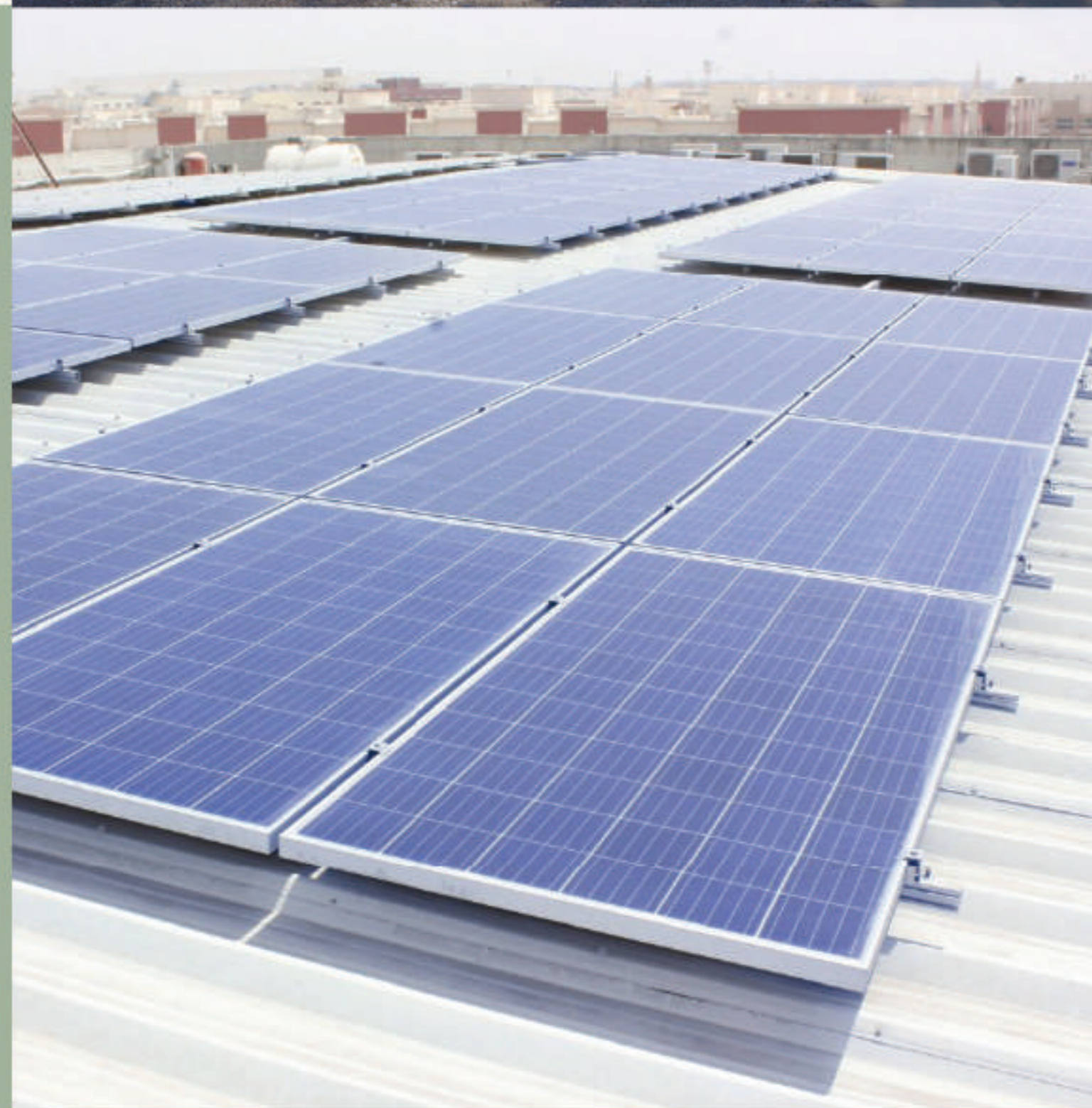
Solar roof Warehouse 0.75 MW
